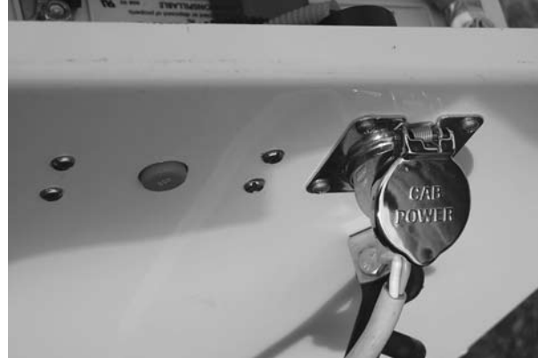
Figure 8 – Shorepower connection installed
